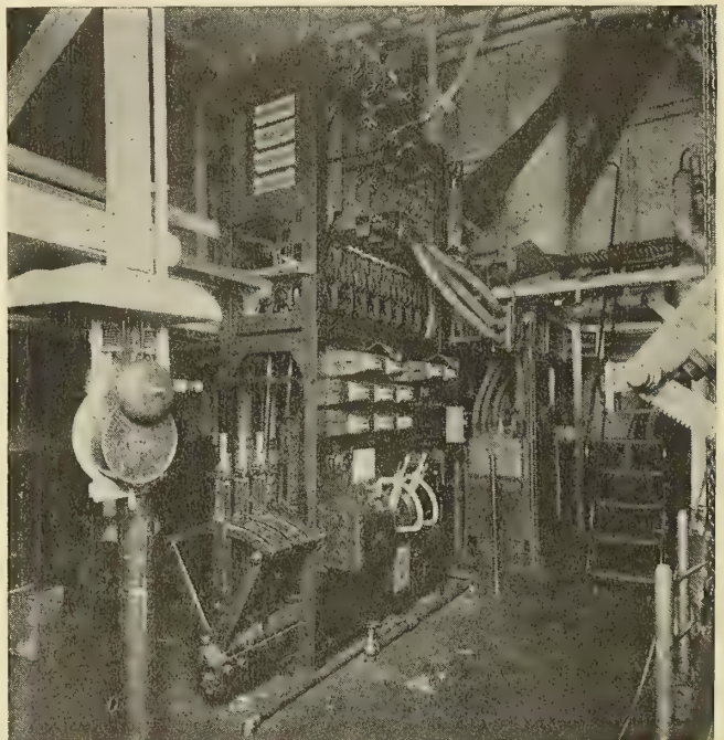
Fig. 9.—General View of Control Board, Showing High-Tension Contactors, Meters, Control Levers and Water Rheostat Which is Connected Into the Secondary Circuit of the Phase-Wound Rotor During Starting and Reversing Operations
